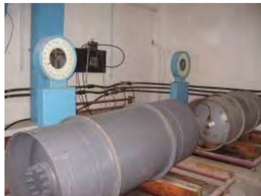
Figura 2.10-22: Echipament de clorinare
