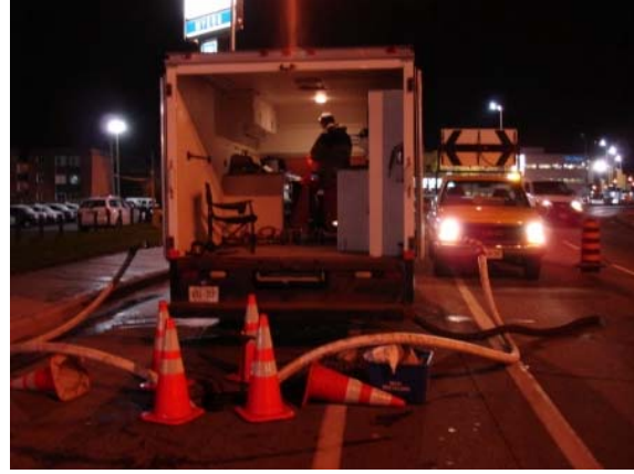
Figure 2: Above ground water supply bypass
