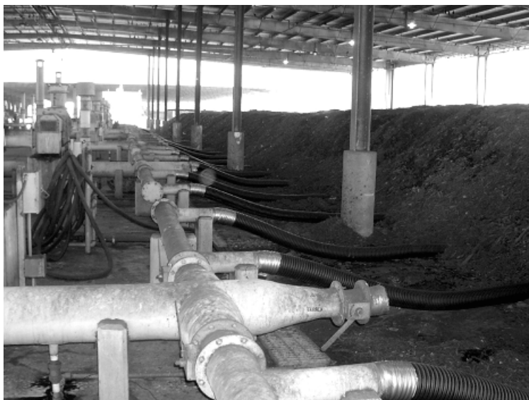
Figure 7.21 View of compost pile and aeration system.
