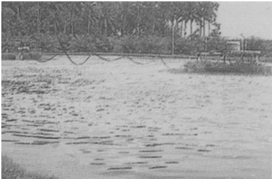
Figure 4.8 An aerator system installed to accelerate BOD reduction at the aerobic pond. (Courtesy of Malaysian Palm Oil Board.)
