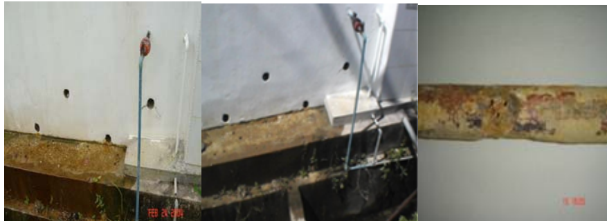
Figure 6 Leaking service pipes
