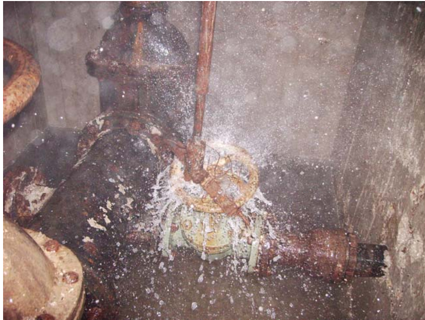
Figure 6: Location of leaks
